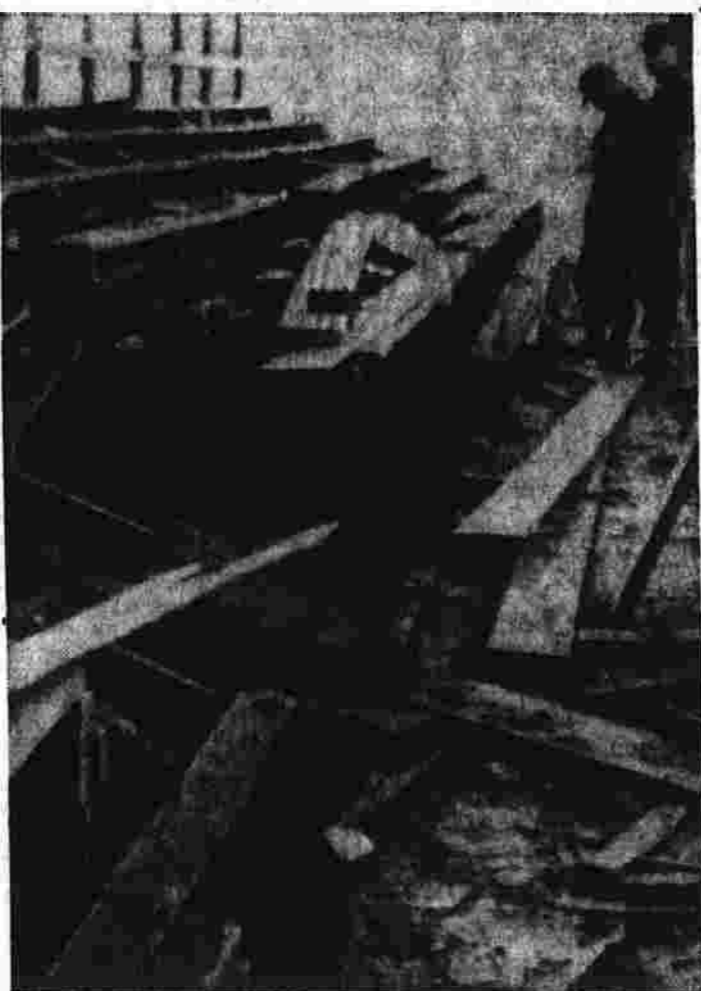
Damage to bleachers in Saigon stadium
